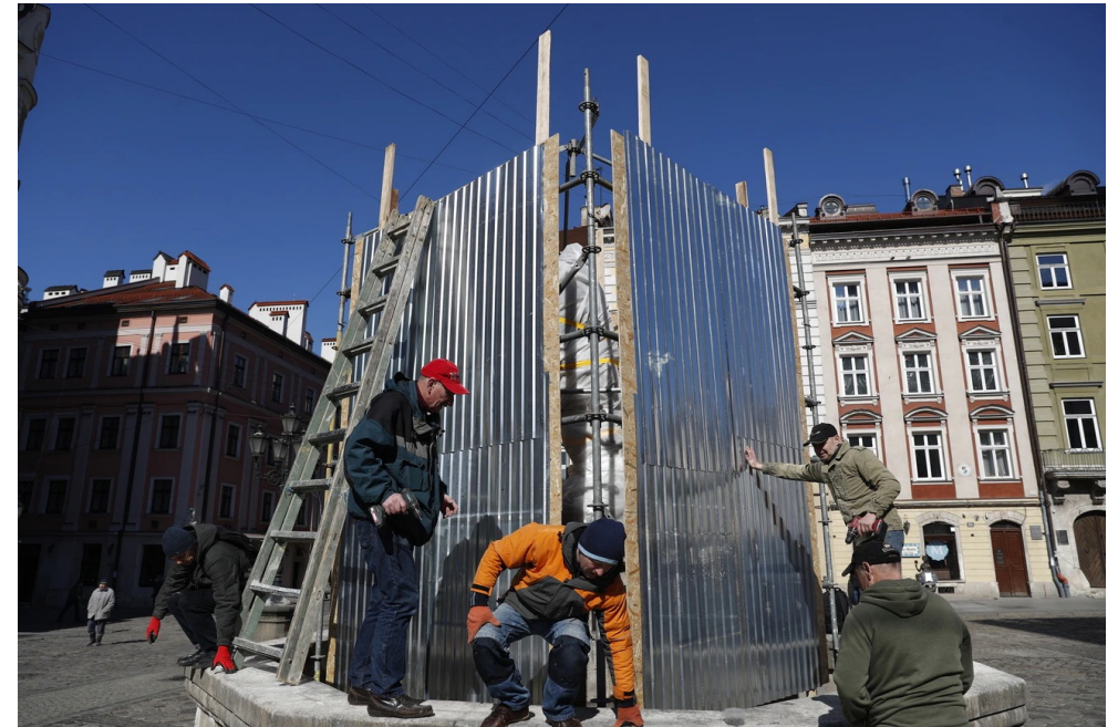
Ukrainian employees build a protection barrier around a historical statue in the centre of Lviv, Ukraine, on March 17, 2022. Keystone / Atef Safad. Source: www.swissinfo.ch/eng/culture/when-cultural-heritage-becomes-collateral-damage-in-war/47511316
